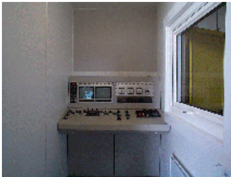
Acoustic Operator Control Room
