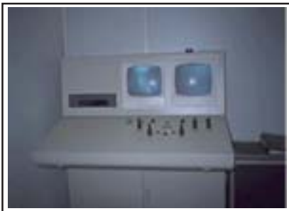
OPERATOR CONTROL CONSOLE
